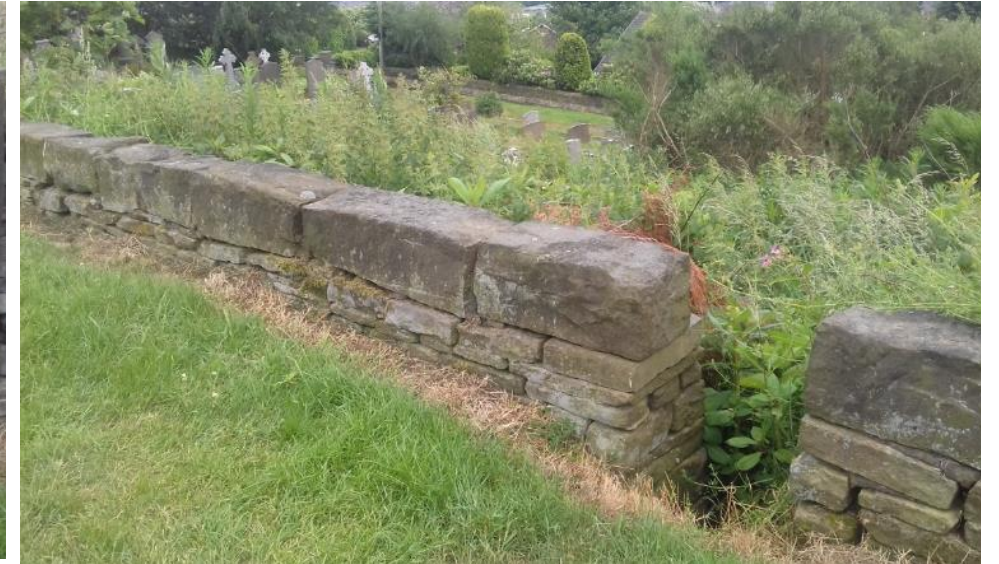
Photo 9: Gap in wall onto 'Moss Side' half way between point A and point E 22/6/2017
